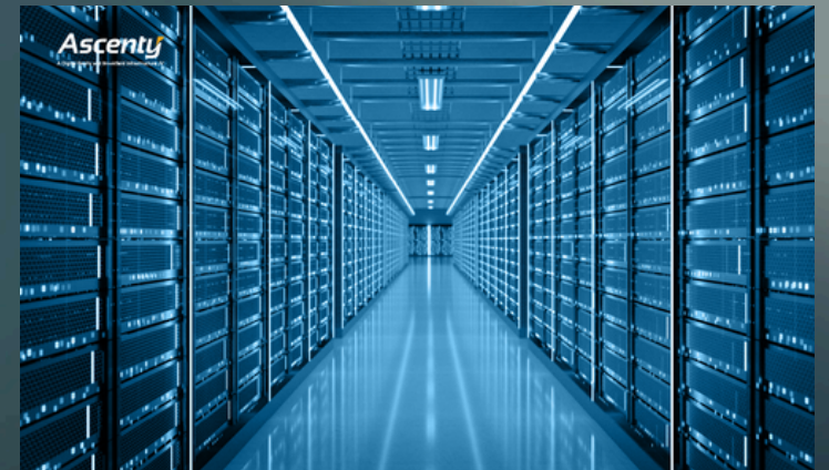
INFRASTRUCTURE OF THE 24 DATACENTERS
